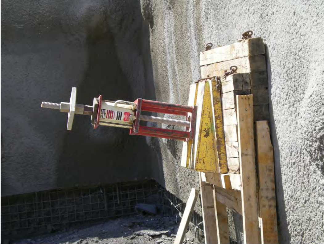
Figure 9.2: Photo. Soil nail load testing setup against shotcrete facing. Photograph courtesy of Schnabel Engineering.
