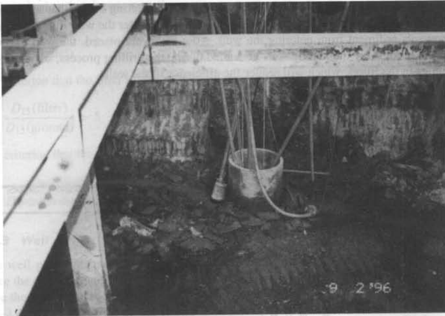
Figure 9.6 Photo of a concrete culvert protecting the side wall of a sump.
