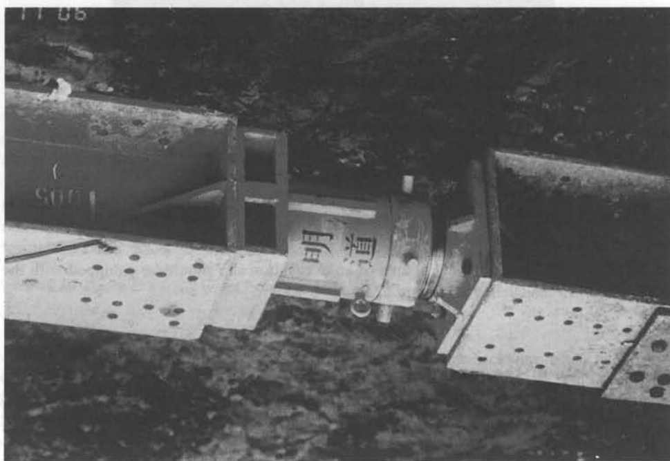
Figure 12.23 Photo of a jack between struts.
