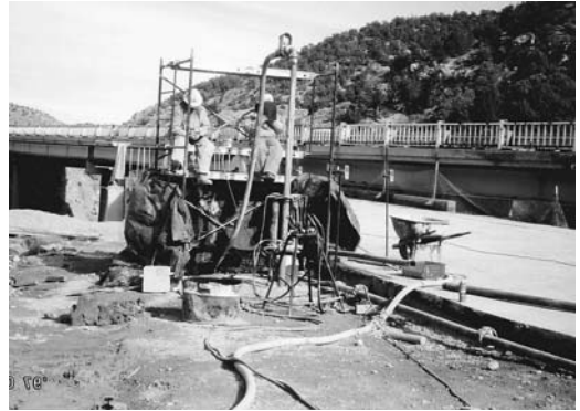
FIGURE 11.51 Access to the header required scaffolding because of 10 ft (3 m) casing lengths.
