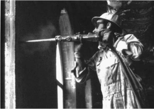
FIGURE 10.19 Drilling with a lightweight pneumatic sinker drill with an integral single chisel-blade bit.
