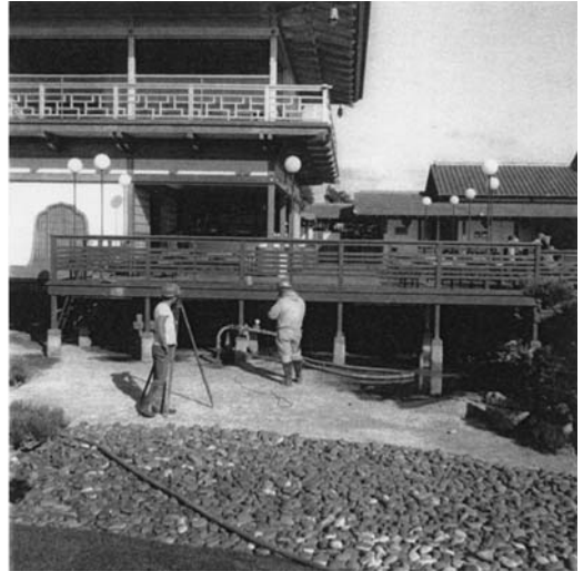
FIGURE 11.18 Compaction grouting of backfill to correct the settlement of a pond liner.
