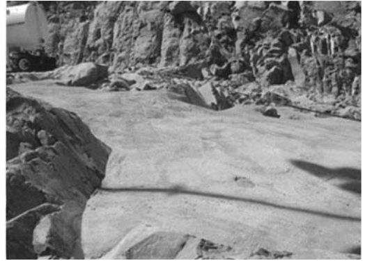
FIGURE 12.12 Depressions in the rock can be filled with dental concrete to provide a relatively smooth surface.
