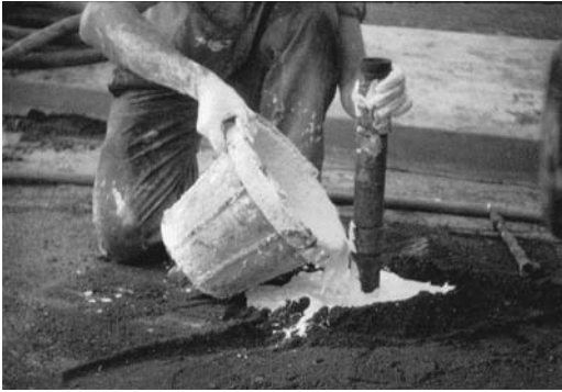
FIGURE 10.34 Encased standpipes must be set precisely to ensure proper trajectory of the drill hole.
