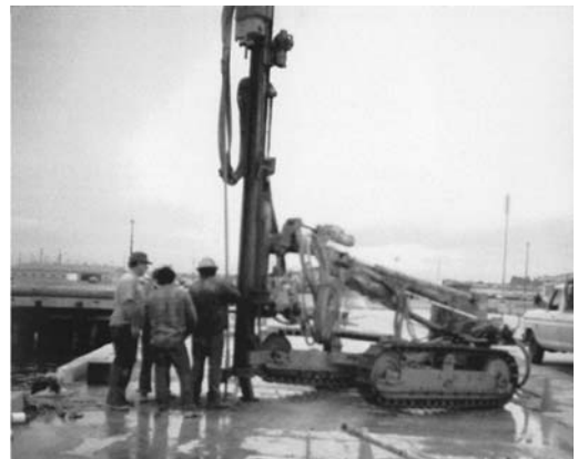
FIGURE 30.8 Air track drills are very maneuverable and provide considerable reach beyond tracks.
