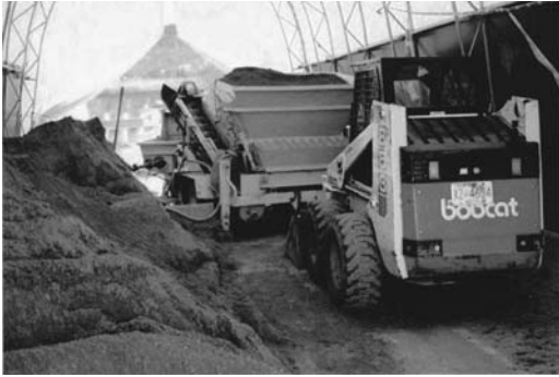
FIGURE 11.33 Aggregate was supplied to the mixer by skid steer loader in the shelter.
