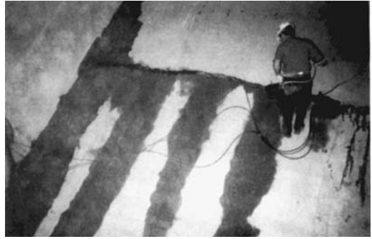
FIGURE 17.1 Apparent leaks in horizontal joints can be deceiving.
