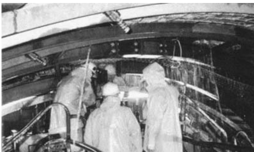
FIGURE 17.7 Severe leaks diminish worker efficiency.
