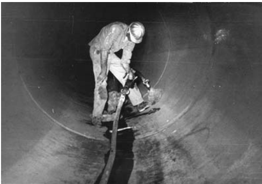
FIGURE 15.6 Improvement of poorly compacted backfill in the lower quadrants of large conduits is a frequent requirement.
