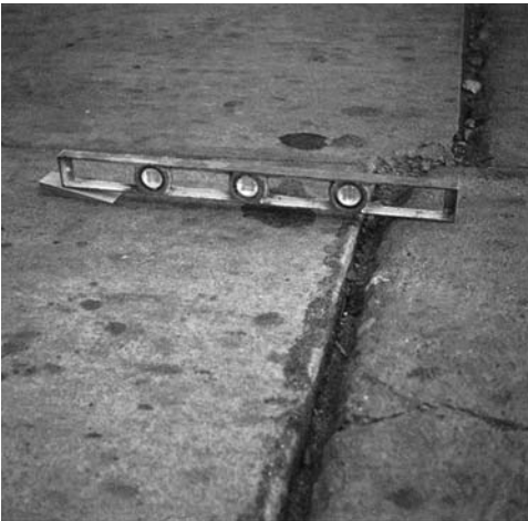
FIGURE 11.10 Differential movement across a crack or joint can easily be observed by the movement of the bubble in a carpenter's level.
