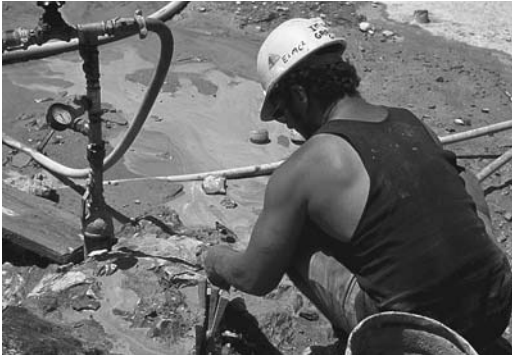
FIGURE 12.23 Surface leaks can sometimes be stopped by caulking with oakum and wedges.
