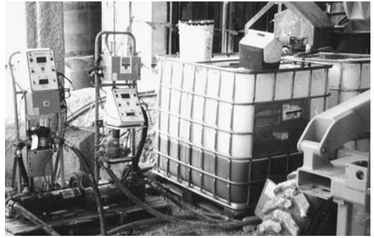
FIGURE 5.11 Bulk supply tanks of liquid admixture with proportioning pumps to facilitate dosing.
