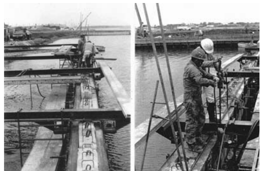
FIGURE 11.37 Test setup with load cells (left). Grout holes drilled with handheld drills (right).
