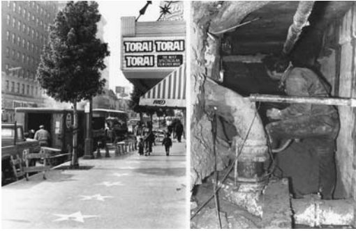
FIGURE 20.7 A broken water main under the walk (left) caused a cavernous void (right).
