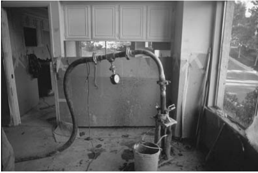
FIGURE 11.44 Knockdown cardboard cartons were used for additional protection of lower portions of the walls.
