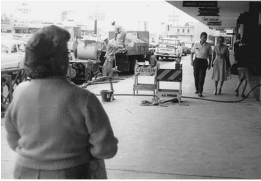
FIGURE 11.17 Loose backfill behind the basement wall in a shopping center being grouted.
