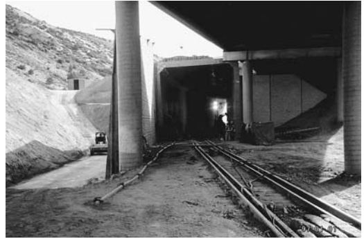
FIGURE 11.48 The left side of the tunnel settled as much as 8 in. (203 mm).
