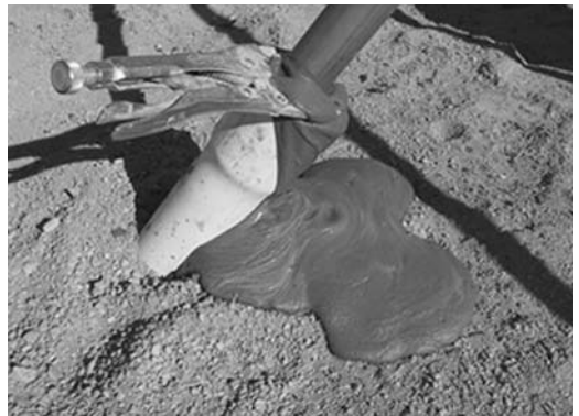
FIGURE 12.20 Grout bypassing the packer sometimes is not discovered until it exits at the hole collar.
