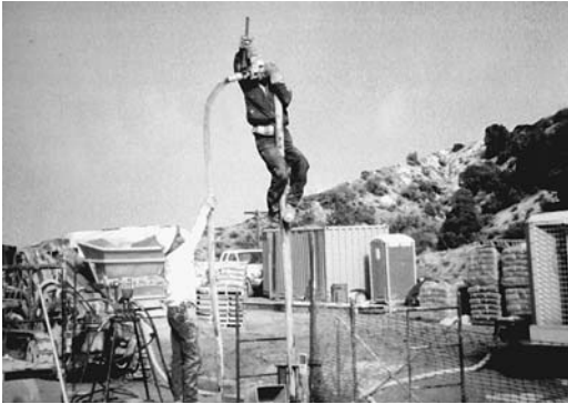
FIGURE 11.3 Acrobatic skills are required of workers when no means of reaching connections are provided.
