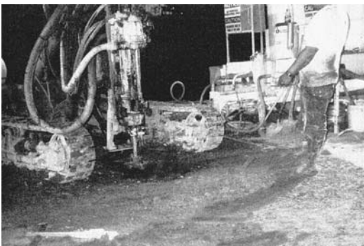
FIGURE 10.32 Failure to use a wash T or other device leads to a messy operation.
