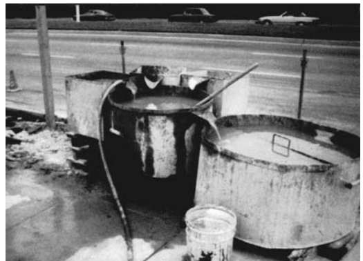
FIGURE 10.30 Settling tanks used to aid separation of drill cuttings.
