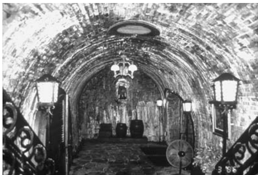
FIGURE 17.14 Excessive seepage forced the closure of museum.
