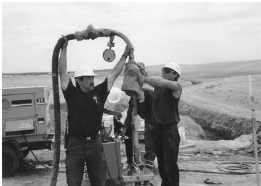
FIGURE 11.26 Casing lengths of 3 ft (0.9 m) are easy to remove from the ground level during withdrawal.
