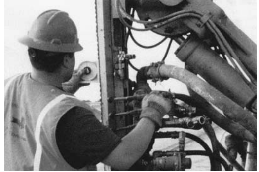
FIGURE 10.36 Driller using a spirit level to plumb the drill mast prior to production drilling.
