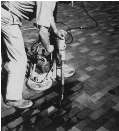
FIGURE 10.23 Removal of a core of the ceramic surface, which will be replaced upon completion of the grouting.
