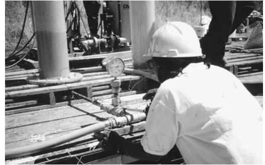
FIGURE 5.10 Injection pressure is controlled through manipulation of valves at the grout header.
