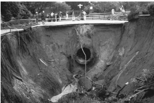
FIGURE 20.1 Sinkhole resulting from loss of ground during underlying tunneling.
