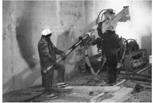
FIGURE 18.10 Frozen grout in rigid delivery pipes had to be drilled out.
