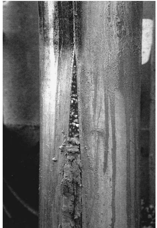
FIGURE 9.9 Vertical split in casing was first detected by a sudden drop in pressure.
