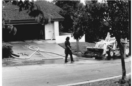
FIGURE 11.46 The work area was washed down at the end of each shift.
