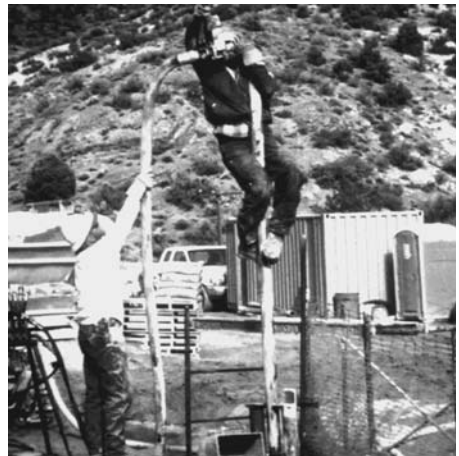
FIGURE 28.4 Long casing joints made breaking precarious and falling header was often damaged.
