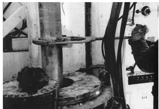
FIGURE 30.14 Welded casing is easily broken with pipe cutter on removal.
