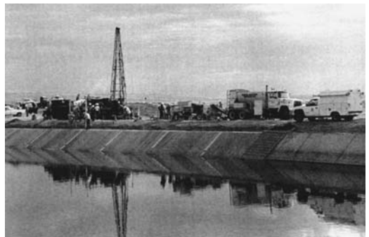
FIGURE 11.27 Overall view of the work area. Canal operations are maintained but at a reduced level.
