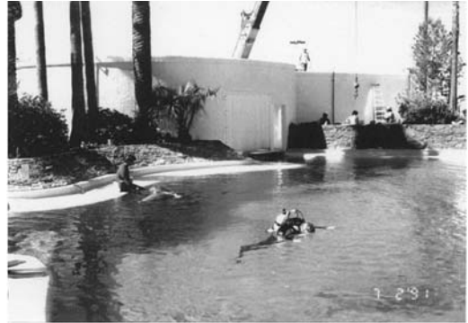
FIGURE 17.17 Dolphin pond was losing 3000 gal of salt water per hour due to leakage.
