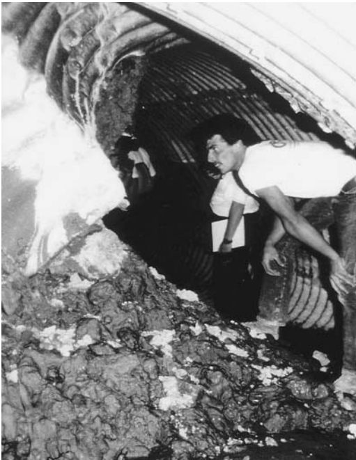
FIGURE 9.10 This culvert was badly distorted and contained a massive amount of grout.
