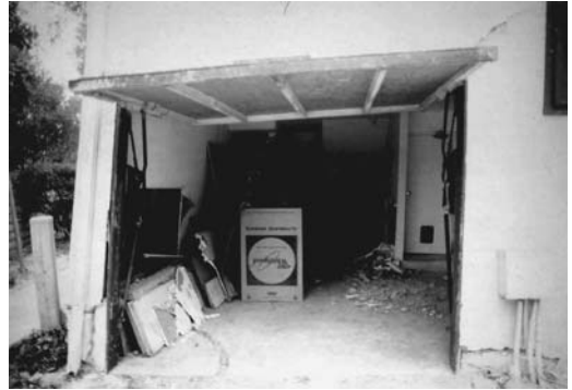
FIGURE 2.23 Wall laterally displaced several inches during blowout of adjacent slope.
