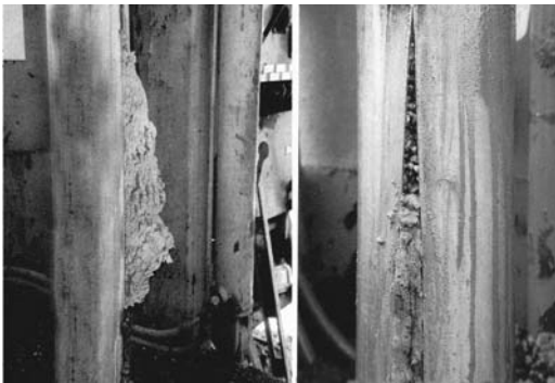
FIGURE 11.5 Fin of grout forced out of split casing (left). Gravel forms a plug where split is less than about 3/4 in. (19 mm) (right).
