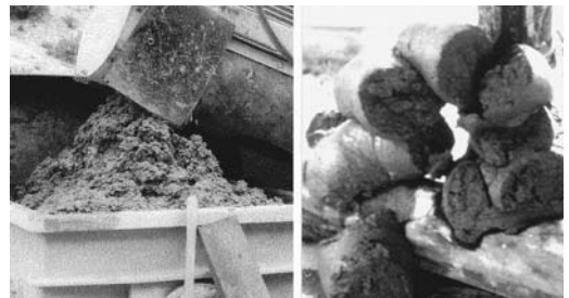
FIGURE 11.6 Rough texture of good-quality grout falling from mixing auger (left). Extruded grout should break off with rough-textured face (right).
