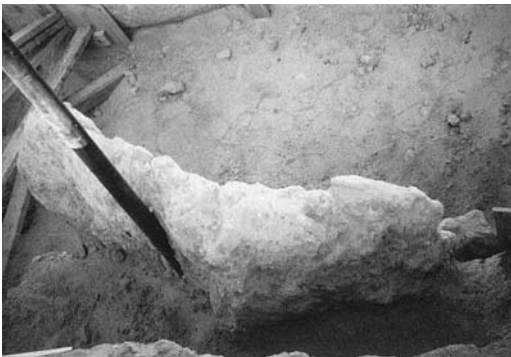
FIGURE 2.15 F grout mass exhibits long, thin wings typical of uncontrolled hydraulic fracturing.
