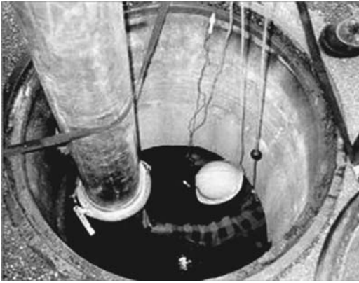
FIGURE 15.1 Oftentimes required ventilation ducts make restricted access even more cramped.
