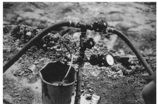
FIGURE 2.2 Grout header containing regulating valves for circulating system.
