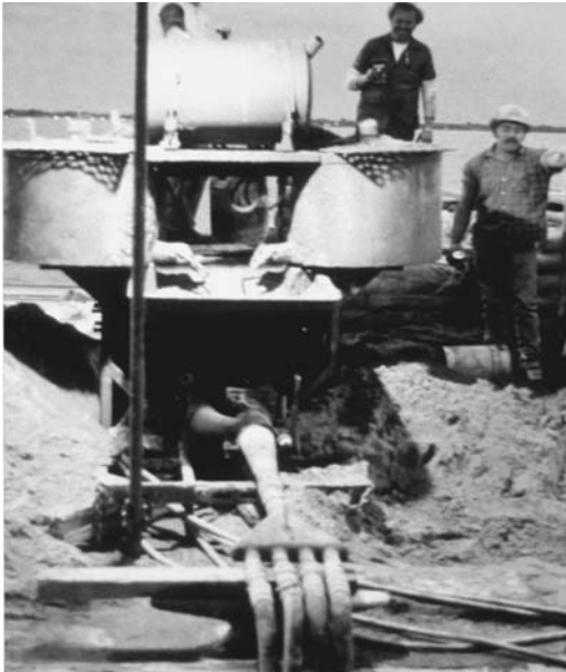
FIGURE 19.20 Grout pump fed common manifold that led to four separate injection lines.
