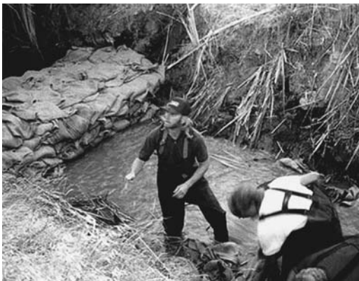
FIGURE 20.4 A sandbag “chimney” will reduce the leakage head and contain escaped grout.
