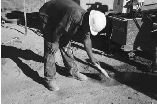
FIGURE 11.16 A worker sweeps the ground so as to be able to see any micro-cracks that develop.
