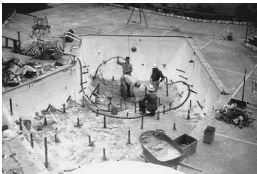
FIGURE 38.3 A swimming pool is filled with muddy water that was squeezed out of fill soil during grouting.
