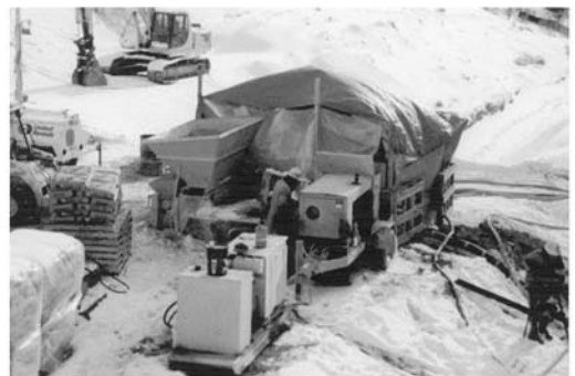
FIGURE 18.2 Makeshift shelter protects the operator but not the equipment.
