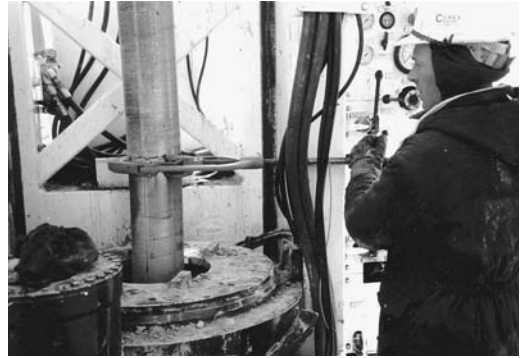
FIGURE 11.29 With rotation supplied by a drill rig, a pipe cutter is used to break joints during withdrawal.
