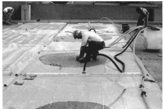
FIGURE 2.32 Vacuum grouting used to fill fine crack network in a parking deck slab.
