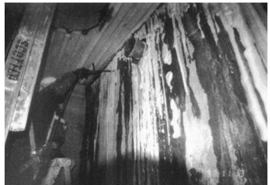
FIGURE 7.13 Spills of hydrophilic urethane are unsightly and stick tenaciously to any surface.
