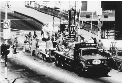
FIGURE 19.15 Grout plug is cautiously placed as firefighters stand by with hoses ready for action.
