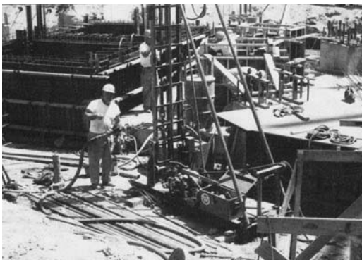
FIGURE 30.4 Custom-built rig is driven by large piston air motor and air-powered winches.
