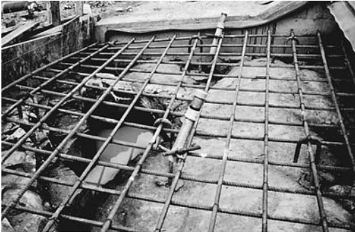
FIGURE 12.13 Grouted anchor rods secure this reinforced grout cap to the rock surface.
