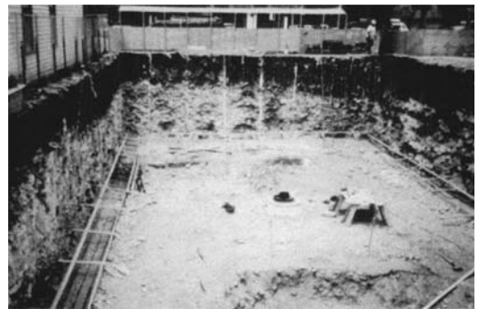
FIGURE 1.4 Solidification of granular soil facilitates shoring and provides soil retention during construction.
