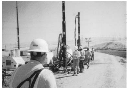
FIGURE 20.3 A line of grout holes upstream of the leak exit will often intercept the water course.
