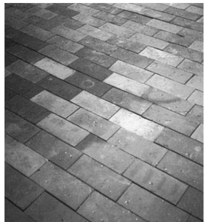
FIGURE 10.24 The surface is restored, with the hole barely visible in the center of the photo.
